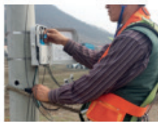
Work Belt on the telephone pole
